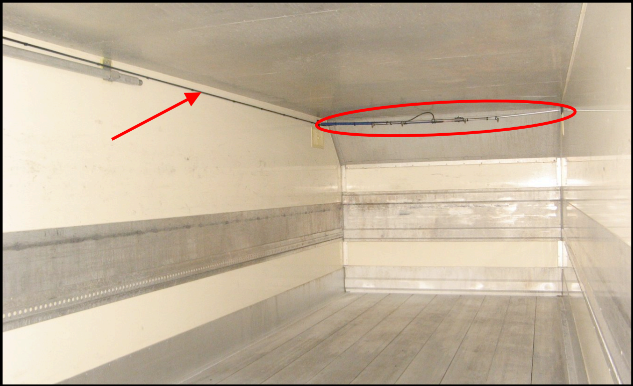
View of the diffusion ramp installed inside and in the back of the truck:
