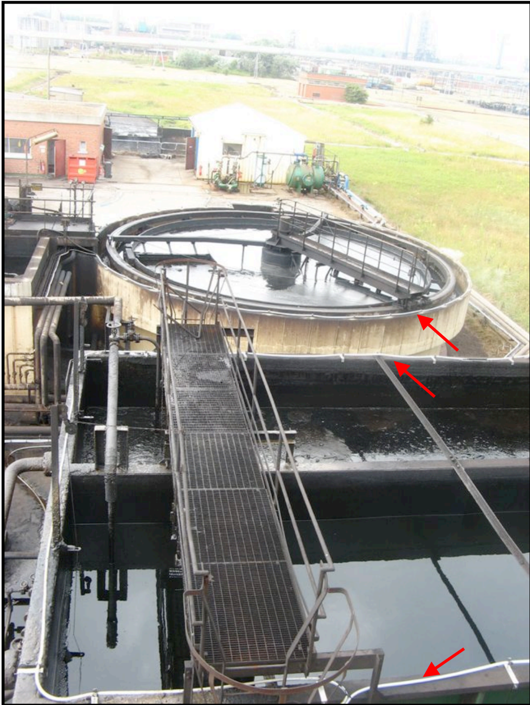
View of the micro-pierced diffusion pipe installed on the tanks border:
