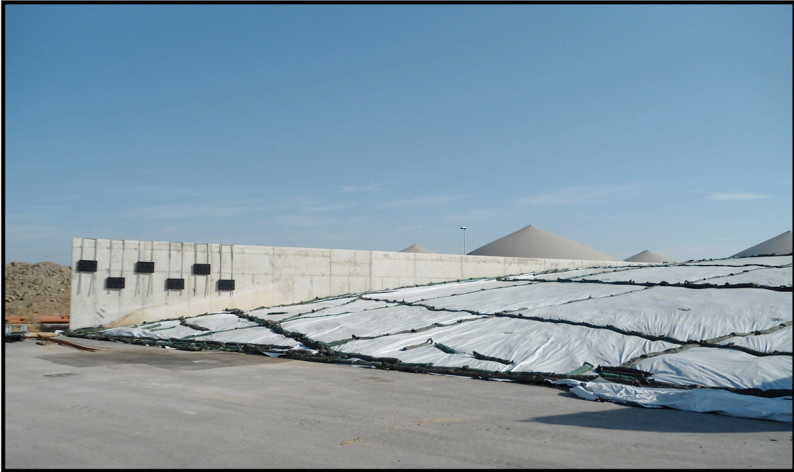
View of the AirForce® 1 installed on the silage boxes:
