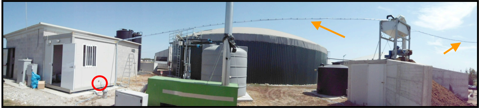
View of the diffusions pipes at the technical room exit going towards the zone 1:
