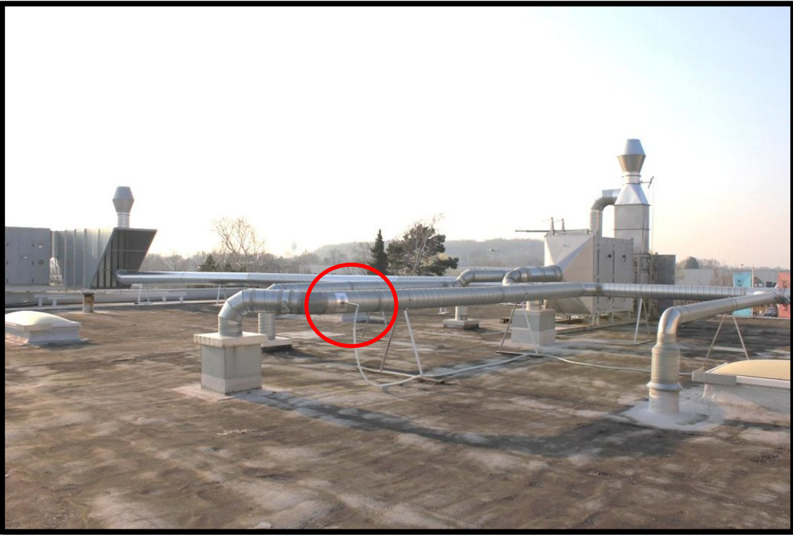
Cheminey's treatment 1: 18.000m 2 /h :
