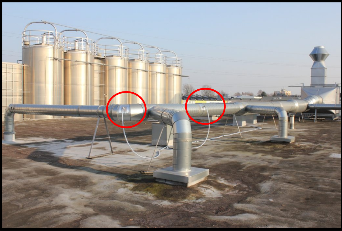
Cheminey's treatment 2: 25.000m 2 /h:
