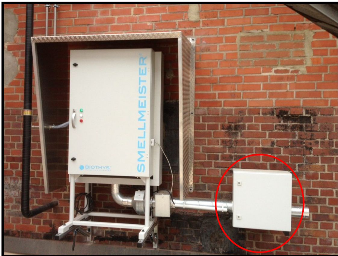
Fresh air heating (without pollution)
